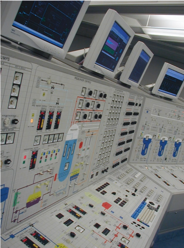
Fig. 1.1 Part of a PWR control room
